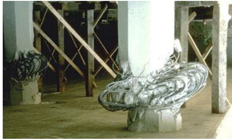
← Buckling of freeway support columns, San Fernando Valley
