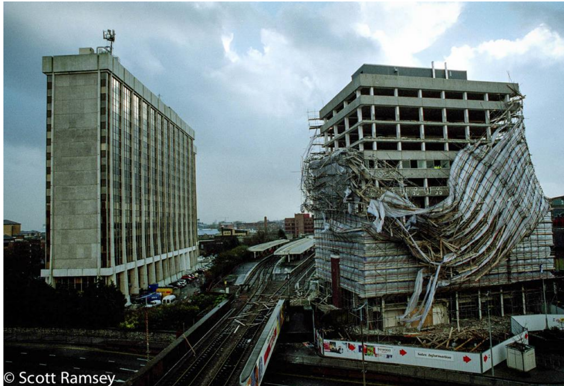
Building damage due to high wind -Cardiff, Wales-
