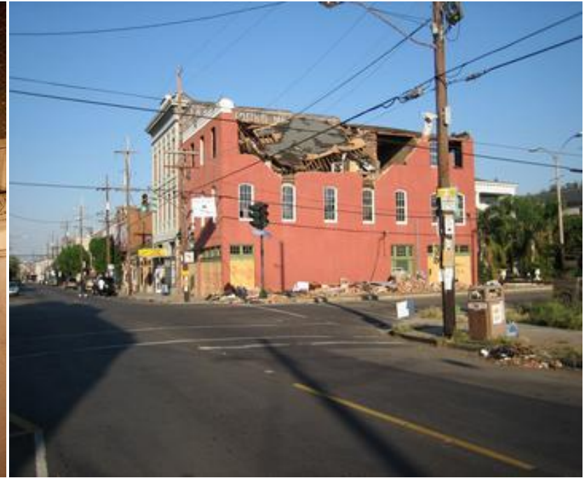
Building failure due to high pressure wind from Hurricane Katrina
